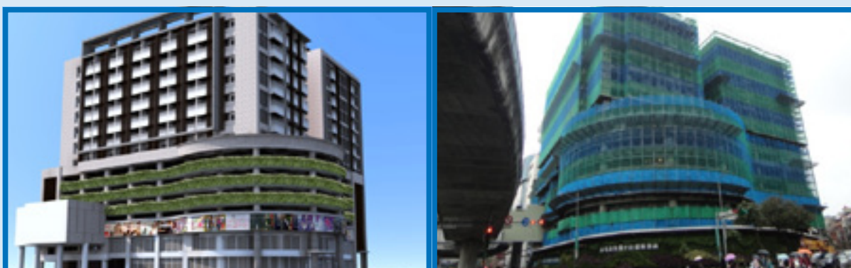
Rendering of Neihu Station (T11) JD project Neihu Station (T11) JD project under construction
