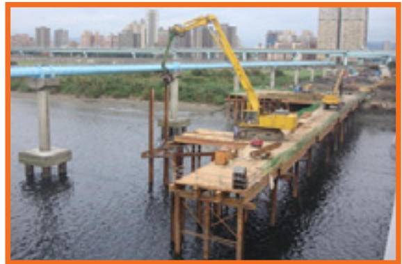
Building a temporary bridge and working platform for the Dahan River section construction
