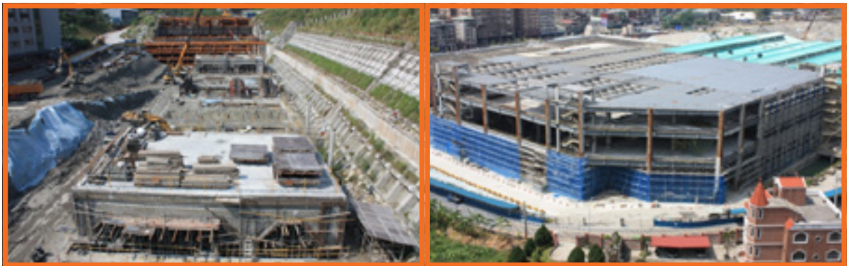
Construction of the extension section tunnel top deck Completed maintenance workshop steel frame
