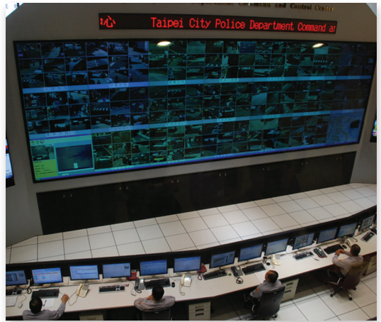
TV wall in the Taipei City Video Surveillance System Center
