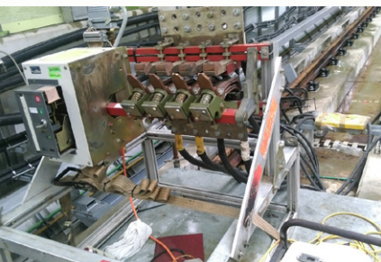
Field integrated short-circuit test of DC System
