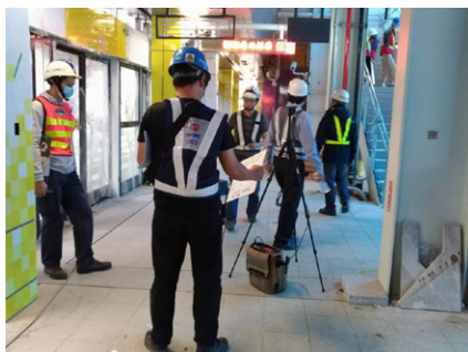
Station Y18 communication public address system acceptance test (COM PA SAT)
