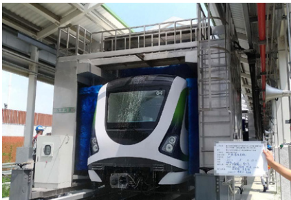
Train washing system site test
