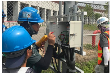
Data Communication System (DCS) subsystem test
