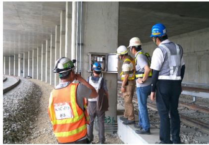
Installation inspection of Communication Systems equipment
