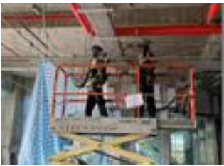
Communication system - cable trough Work and distribution
