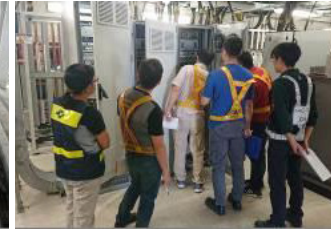
Operation Control, Communication Room equipment handover
