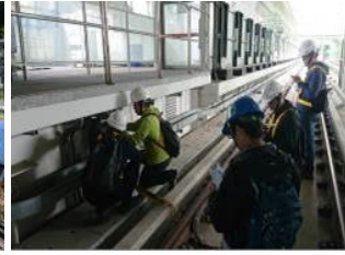
Operation Control, track-side equipment handover
