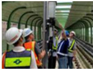
Communication system - handover to TMRT
