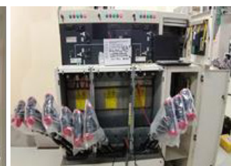
RMU IAT test for substation power supply at Depot station
