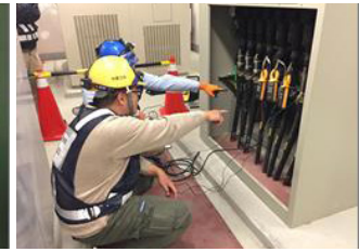
PWR, 22kV cable voltage sensor checks
