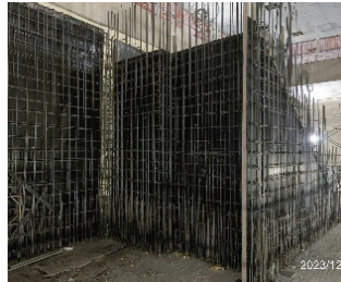
Rebar tying for buttress of escalator from B2 to platform level at Station LG06
