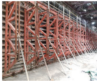
Assembly and installation of the formwork of the concourse side walls at Station LG01
