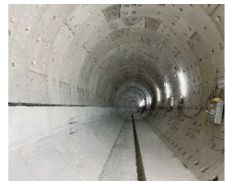
Station LG02-LG03 up track work completed for the walking path in the shield tunnel
