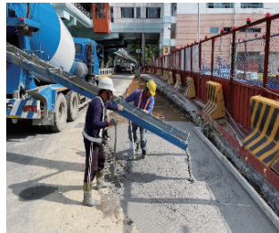
Station Y1 south sidewalk removal work from Maokong Gondola Station to Taipei Zoo Station
