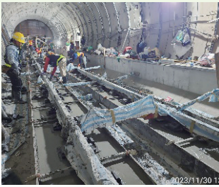
Ballastless bed work for the up track in the tunnel of Xiangshan Station tail track
