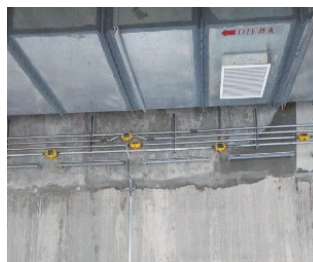
Pipe distribution for track lighting; OTE ventilation pipe work
