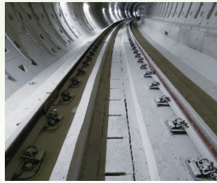
Ballastless bed completion for the down track in the tunnel of Xiangshan Station tail track
