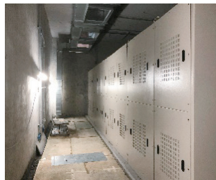
Switchboard placement and installation at low-voltage substation A, Station LG06
