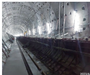
Walking path work inside the shield tunnel between Station LG02-LG03 up track
