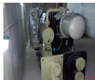
Placement of the water chiller
