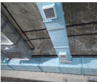
A/C wind pipe work at the platform level
