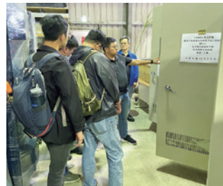
Fifth equipment inspection (electric remote-control system) of contract CR385A
