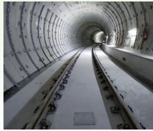
Completion of floating slab track construction and jacking in the tunnel of Xiangshan Station tail track
