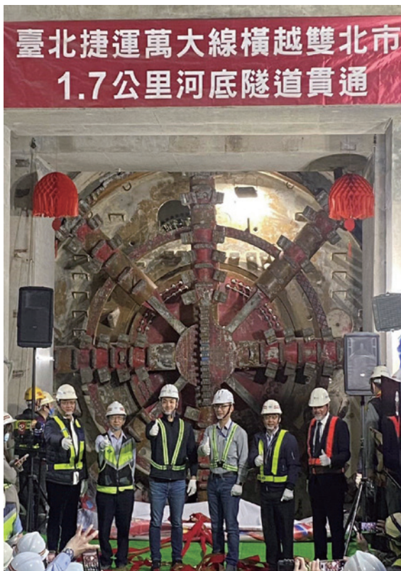
Photo 5: Mayor Chiang Wan-an inspected the up-track tunnel breakthrough construction which traverses the Xindian River from Wanda line Kalah Station to Yonghe Yongping Elementary School Station (March 6)
