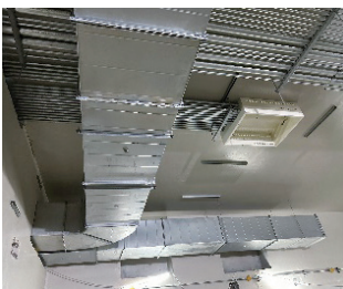
Server room wind pipe and electrical conduit work at the equipment level, Station LG07
