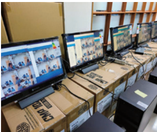
Telecommunication system and CCTV testing at the manufacturing plant
