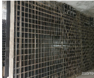
Rebar tying for partition wall at B1 concourse level of Station LG06
