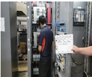
Performance test of the low-voltage switchboard
