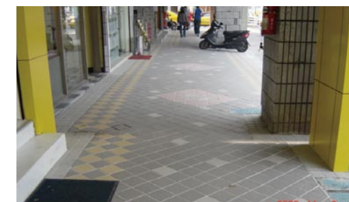
Colonnade leveling of Heping East Road Sec.2 No. 20.
