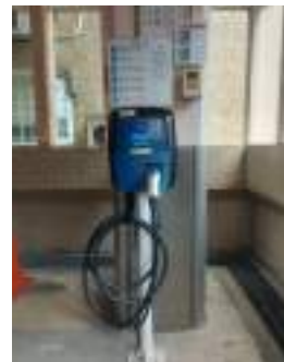
Electric car charging station
