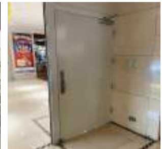
Automatic fire proof steel coiling doors should be cleared in fire proof area
