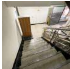
Emergency escape staircase is stacked with items and hinders emergency escape
