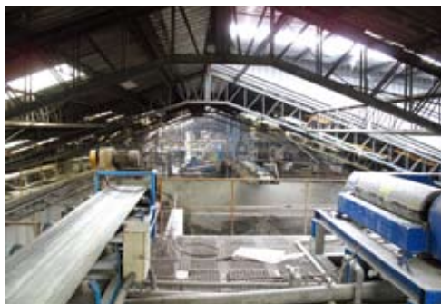
Facilities installed at the Incinerator Bottom Ash Recycling and Reuse Factories.
