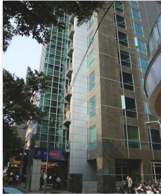
Intense sunset heating on glass curtain wall
