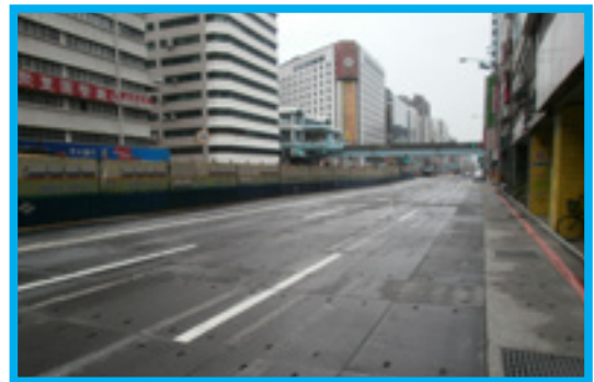
Composite decking without steel rim used in the cut-and-cover area on Nanjing E. Rd.
