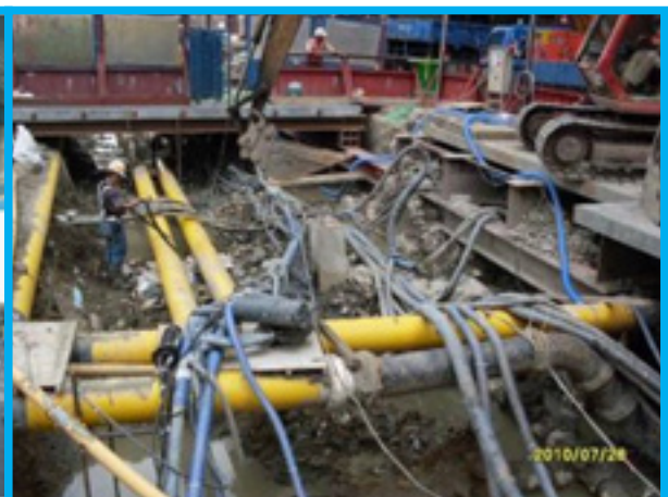
Intricate underground pipeline
