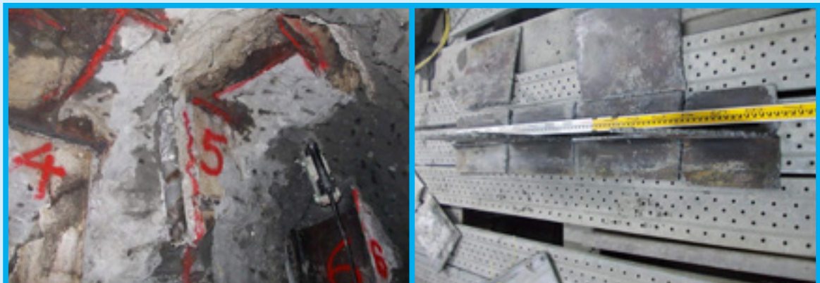
Treatment of group piles beneath the Tacheng Park underground parking lot to allow passage of a shield tunnel between Beimen and Zhongshan stations
