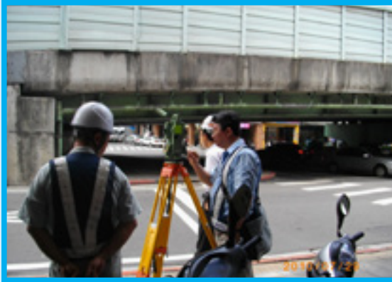
The civil works 6 th site office of DORTS Central District Project Office, detailed design consultants, and contractors jointly conducted on-site surveys and investigation
