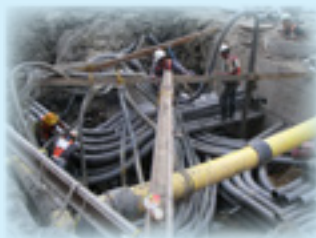
Intricate pipeline beneath Nanjing East and West roads
