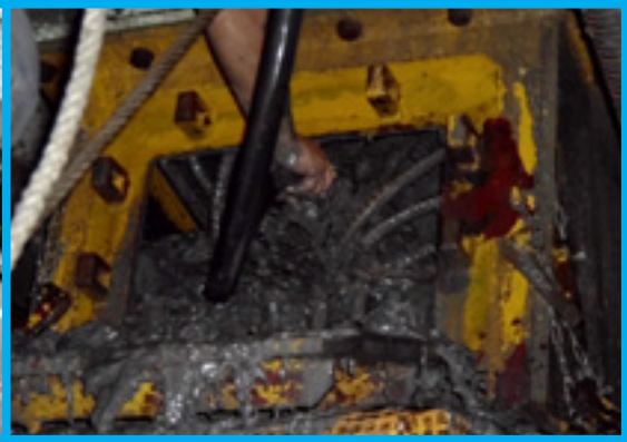
Foundation pile steel bars belonging to the Zhengqi Bridge were excavated through the P0 pump gate
