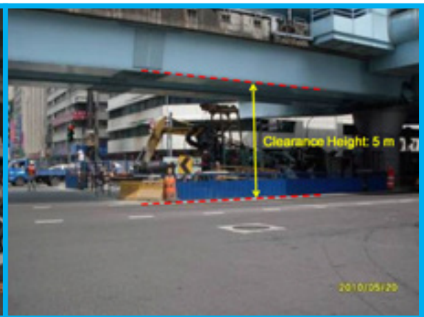
Due to height limitations, the diaphragm wall method was replaced by the reversed circulation pile construction method. Tangent piles, used to facilitate small machines, reduced construction efficiency
