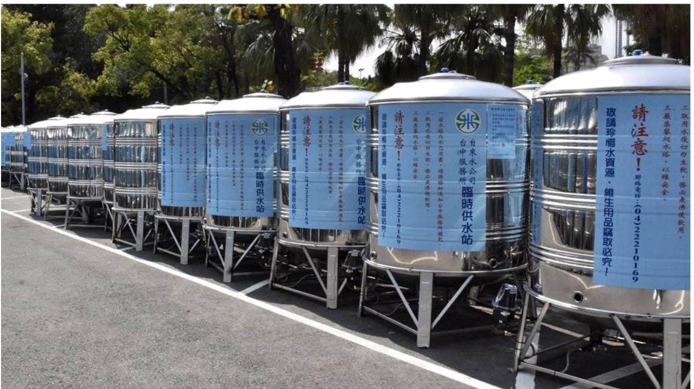
Temporary Water Supply Stations / Source: Water Resources Agency
