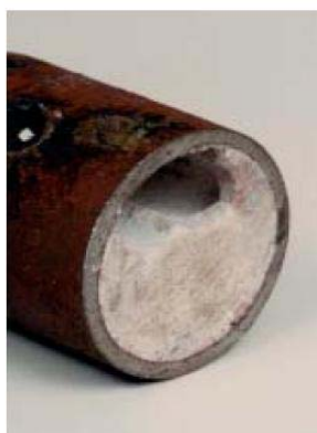
Boiler scale on water side
