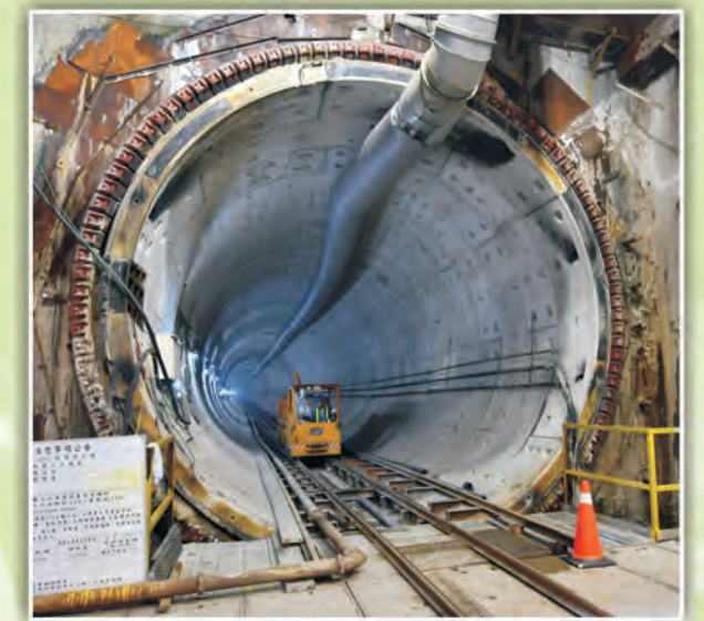
▲ 植物園站潛盾隧道施工 Shield tunneling construction at Taipei Botanical Garden Station
