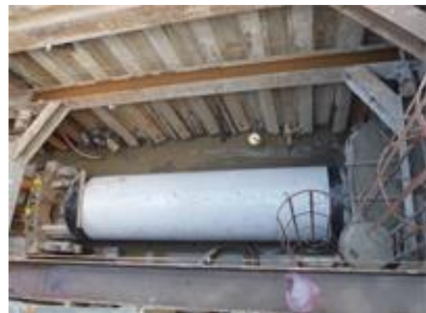
Fig.4 jacking pipe settlement of start shaft
