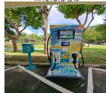
DC快充充電樁
